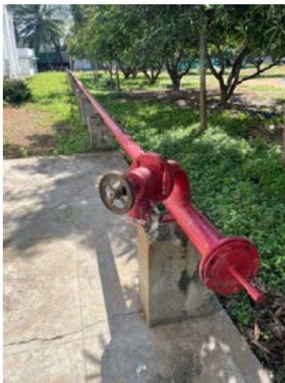
Hydrant at Hostel.JPG
