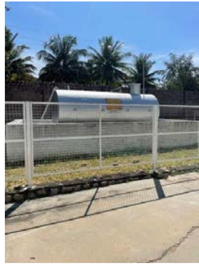
Diesel storage tank as per legal norms.JPG
